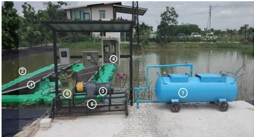
Figure 3.9 Working system and equipment of the 3 kW solar aerator system
